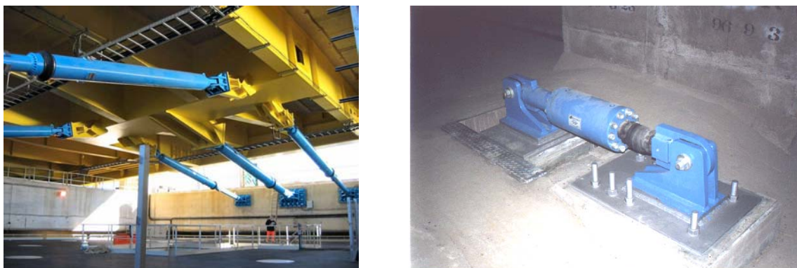
Figure 18 –Installation examples of Italian fluid viscous dampers: in the Rion-Antirion main bridge, Greece (left) and in the Seohae Bridge, Korea (right).
