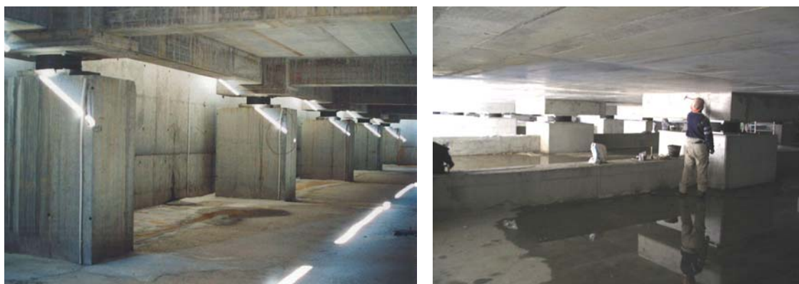
Figure 2 – Elastomeric isolators installed in the Hospitals of Udine (left) and Lisbon (right).
